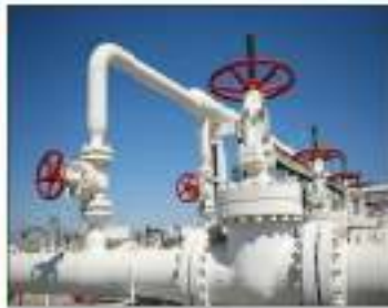
Gas Pipe Lines
